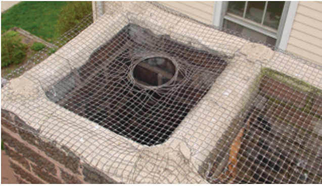
Figure 7. A raccoon made a home in this chimney after breaking through this “home-made” chimney screening. Non-professional screenings also may become packed with snow or ice thereby forcing toxic exhaust gases back into the home.
